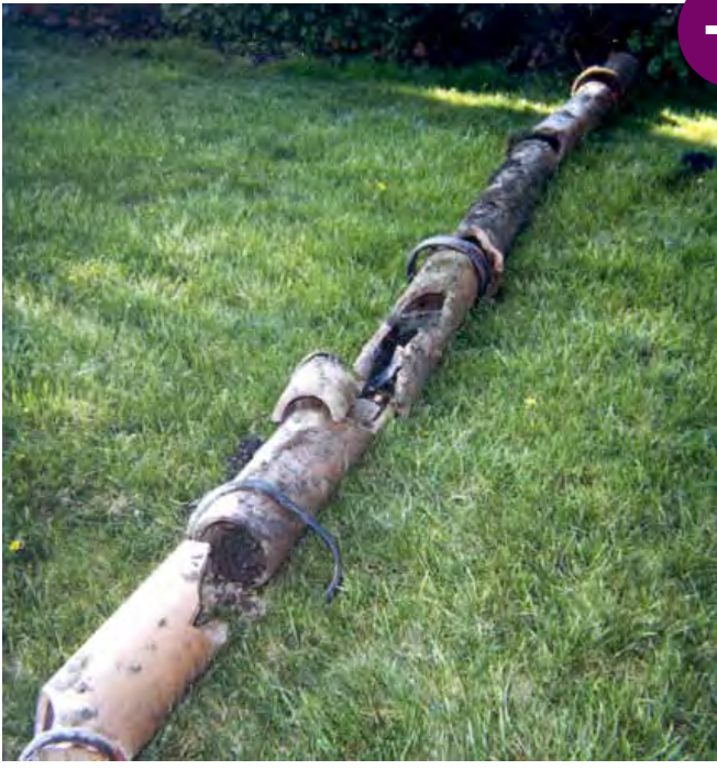
Leaky Lateral Pipe
