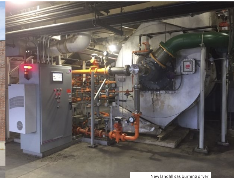
New landfill gas burning dryer
