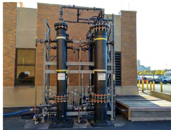
2 Flash Columns 2 Vertical Absorbers Horizontal Absorber in a box
