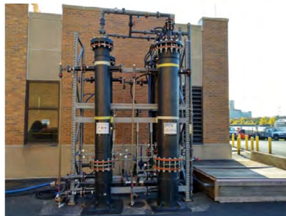
2 Flash Columns 2 Vertical Absorbers Horizontal Absorber in a box
